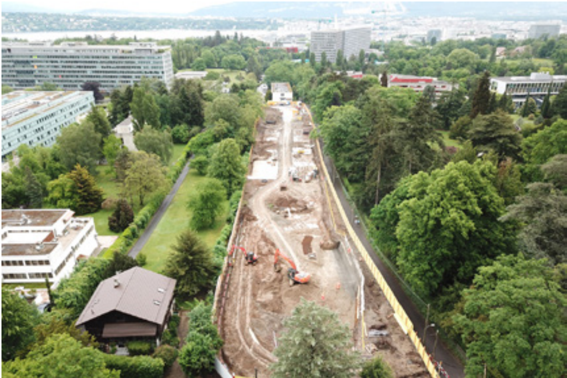
Route de Ferney near WTO, Geneva Construction site of the future Route des Nations
