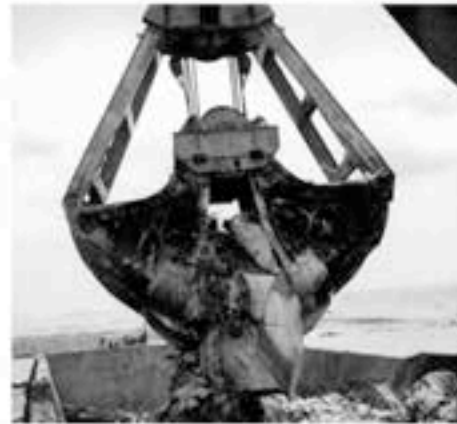
Large clay lumps are taken from the seabed and dumped into construction sites by bottom opening barges.
