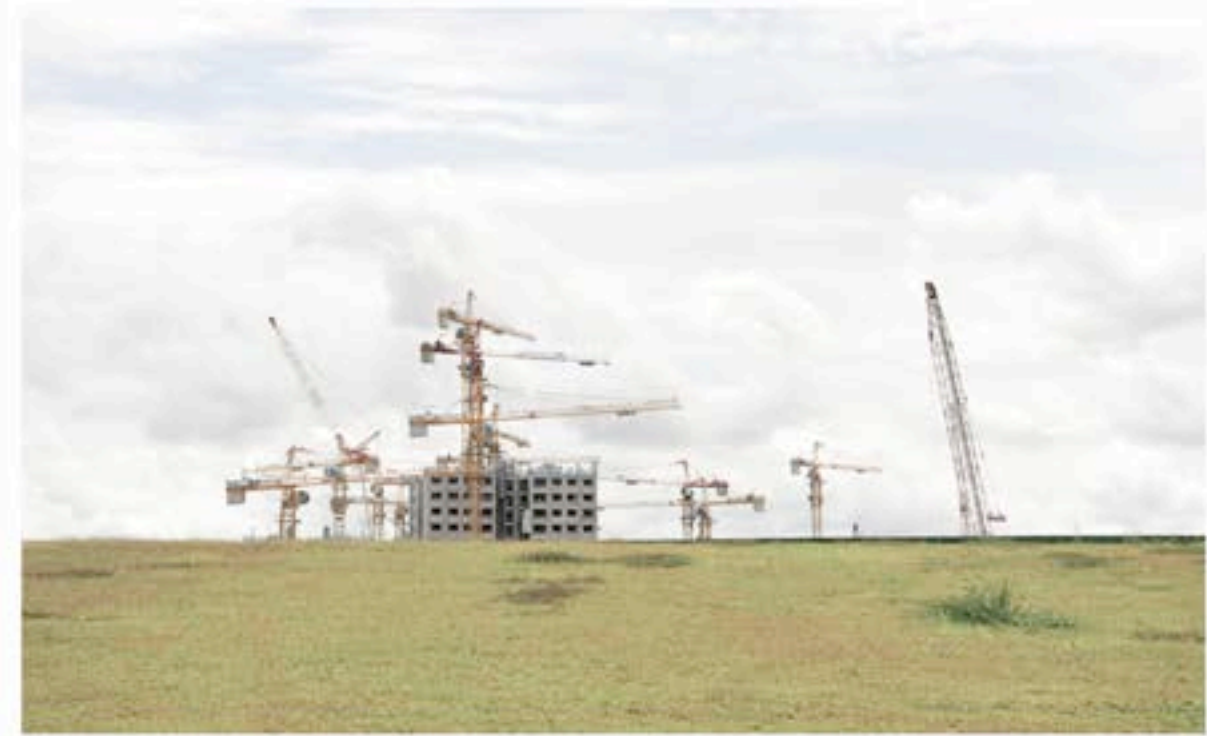
1. Bare field in wait of investors 2-4. City in construction with the green belt already built in the foreground
