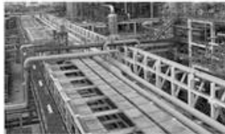
Left: Semboorp Pipeline
